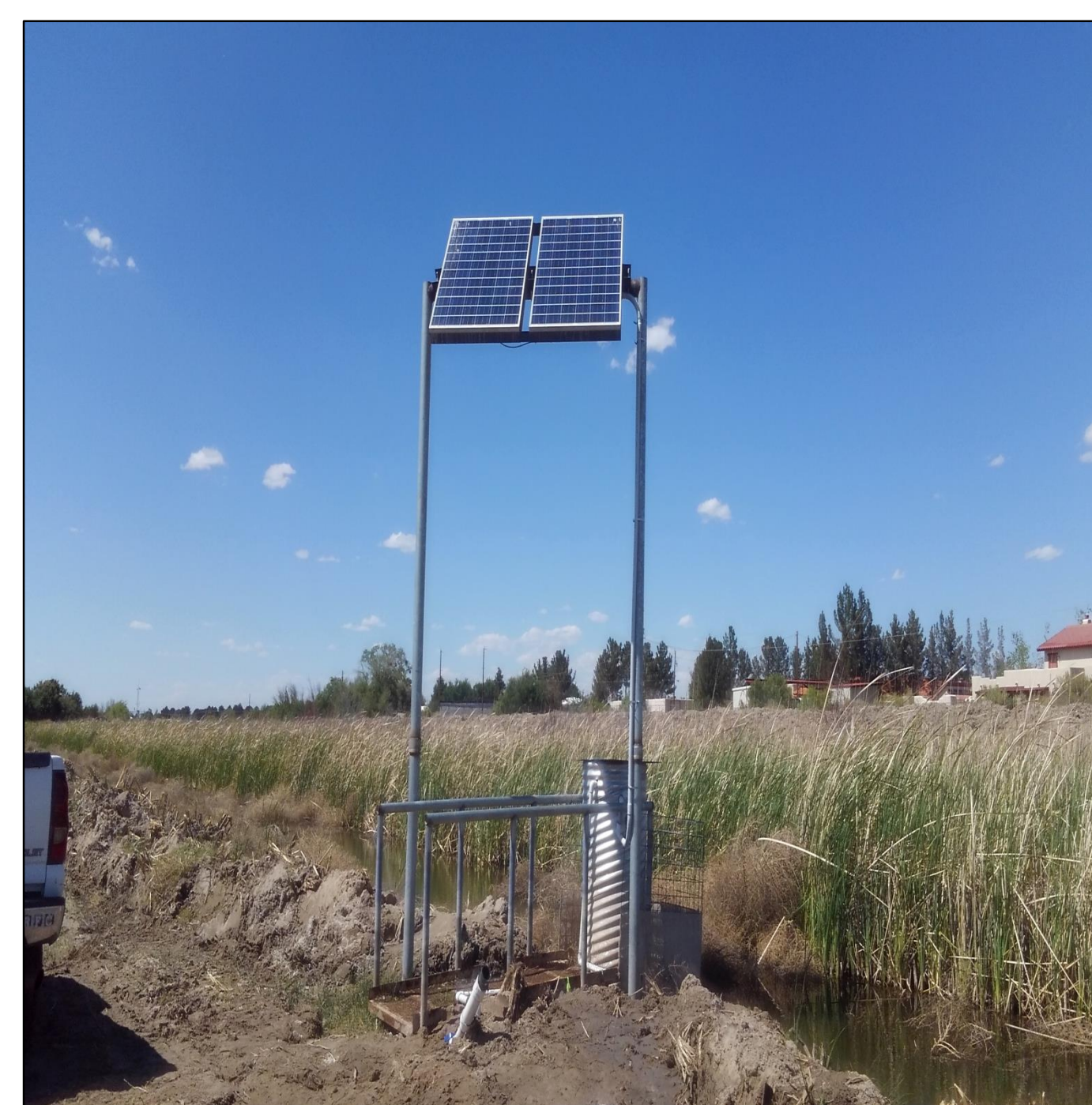
Figure 5. Solar pump used to pump water from Diez Lagos canal.
