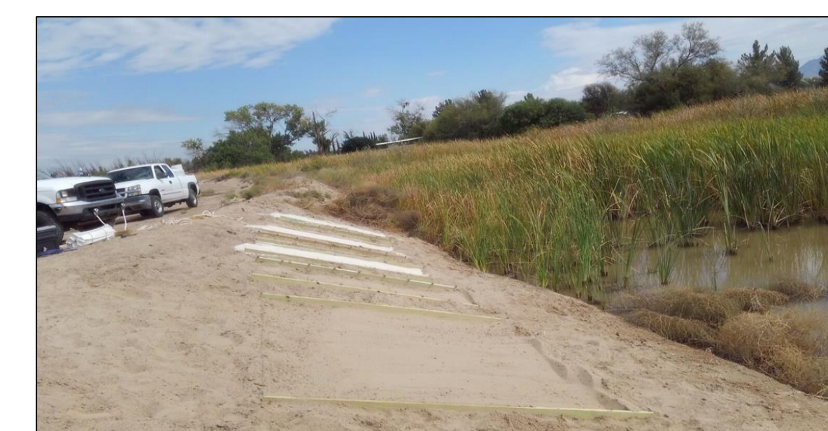
Experimental setup on the embankment of Diez Lagos earth drainage canal at the Sunland Park ReNUWIt Test-Bed
