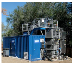
Figure 2. Sequencing-batch membrane bioreactor (SB-MBR) located at the Mines Park testbed.
