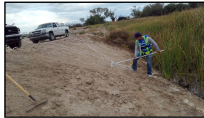
Figure 1. Embankment during cleaning showing sandy soil prone to erosion (side slope: 30 %).
